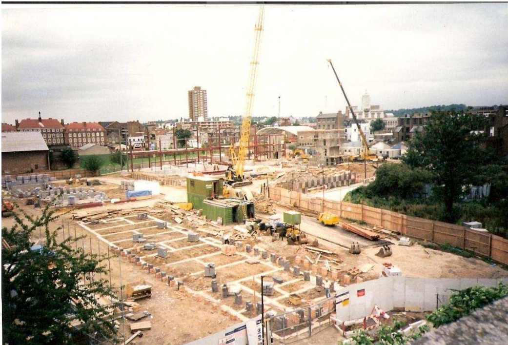
Image 5: Regeneration of the Five Estates. Foundations for the new houses. Photograph by Stacey.
